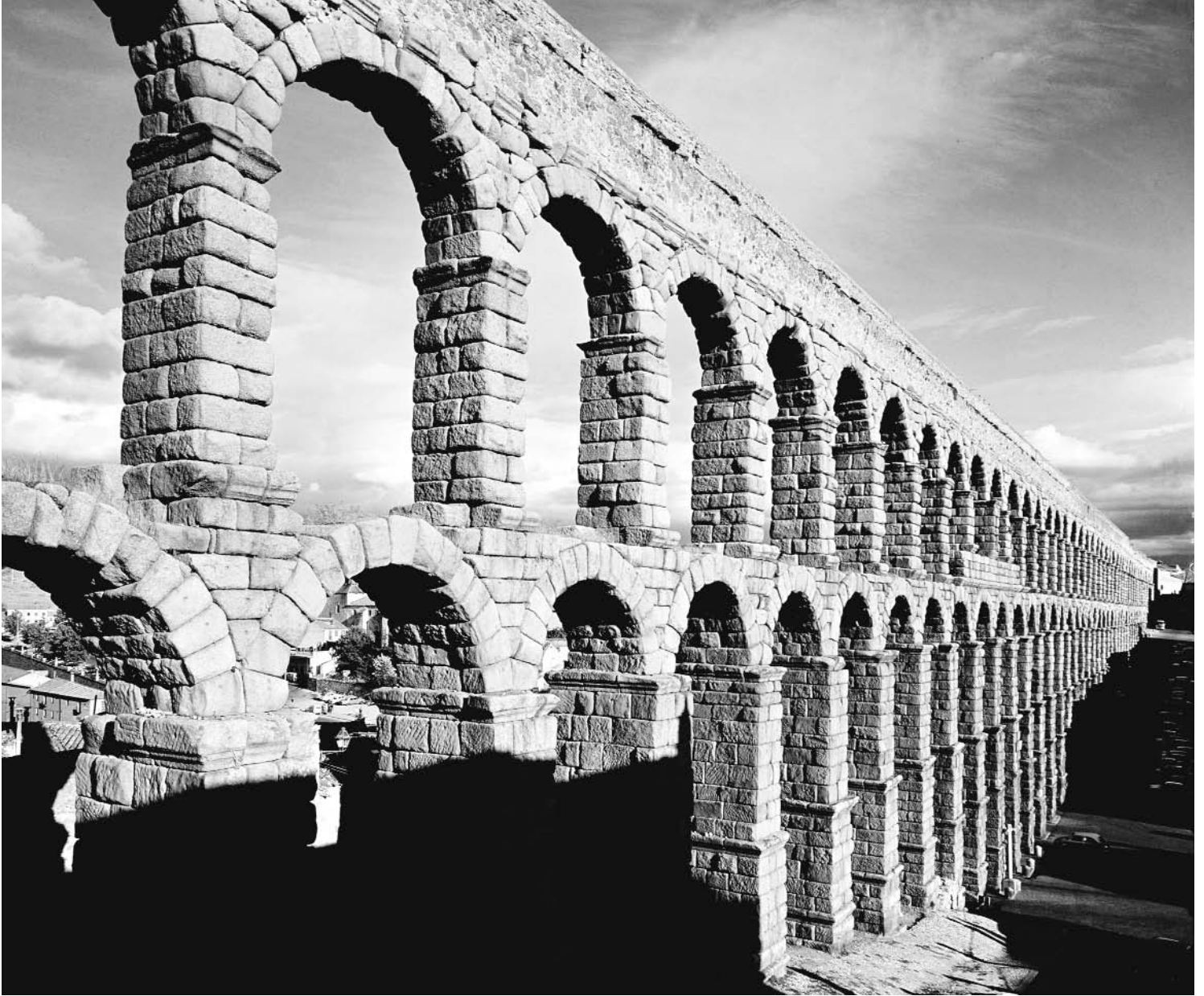
This granite aqueduct in Segovia, Spain, built without mortar or cement, has endured for 2,000 years, but pollution and age are slowly deteriorating it.
