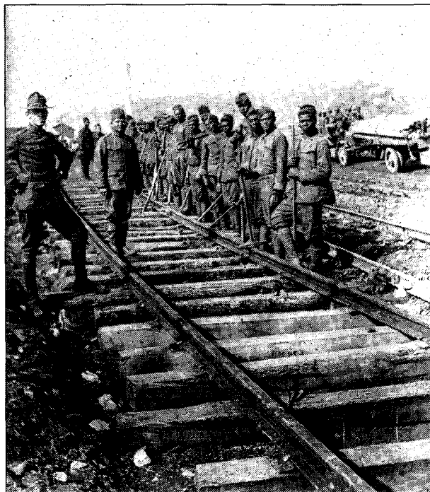
A segregated unit of African-American troops in World War I constructing a railway line from Brest to the front.
