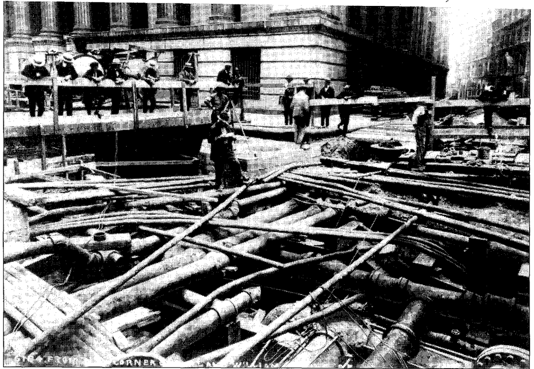
Construction on Manhattan's Wall Street in 1917 revealed a tangle of pipes and conduits—an apt metaphor for cities' efforts to grapple with the infrastructure crisis of the day.
