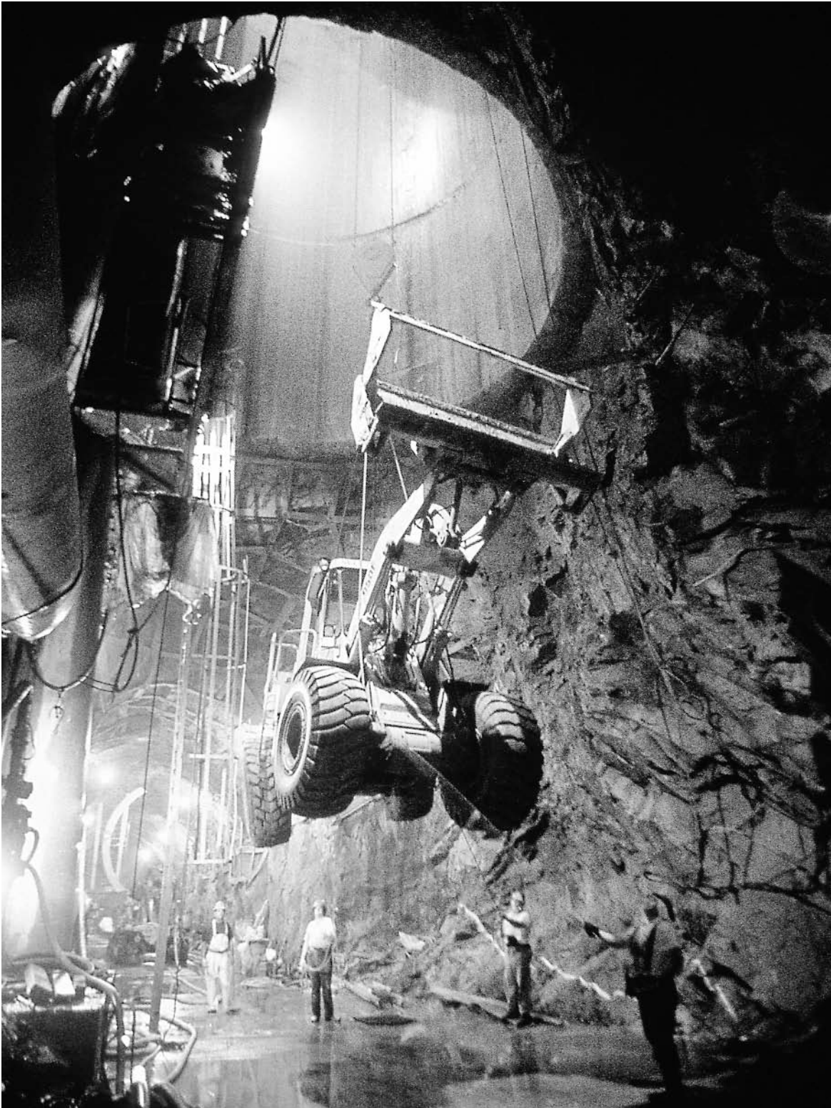
A front-end loader is lowered into a huge water tunnel hundreds of feet below the New York City streets. Begun in 1970, construction will continue until 2020.
