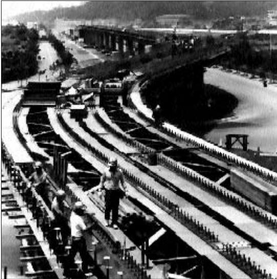
Using some of the wealth generated by the robust economy, the Taiwan government has embarked on an ambitious program to modernize the island's infrastructure.
